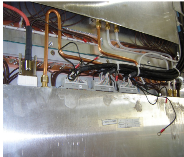
Interconnecting gas and coolant pipes
