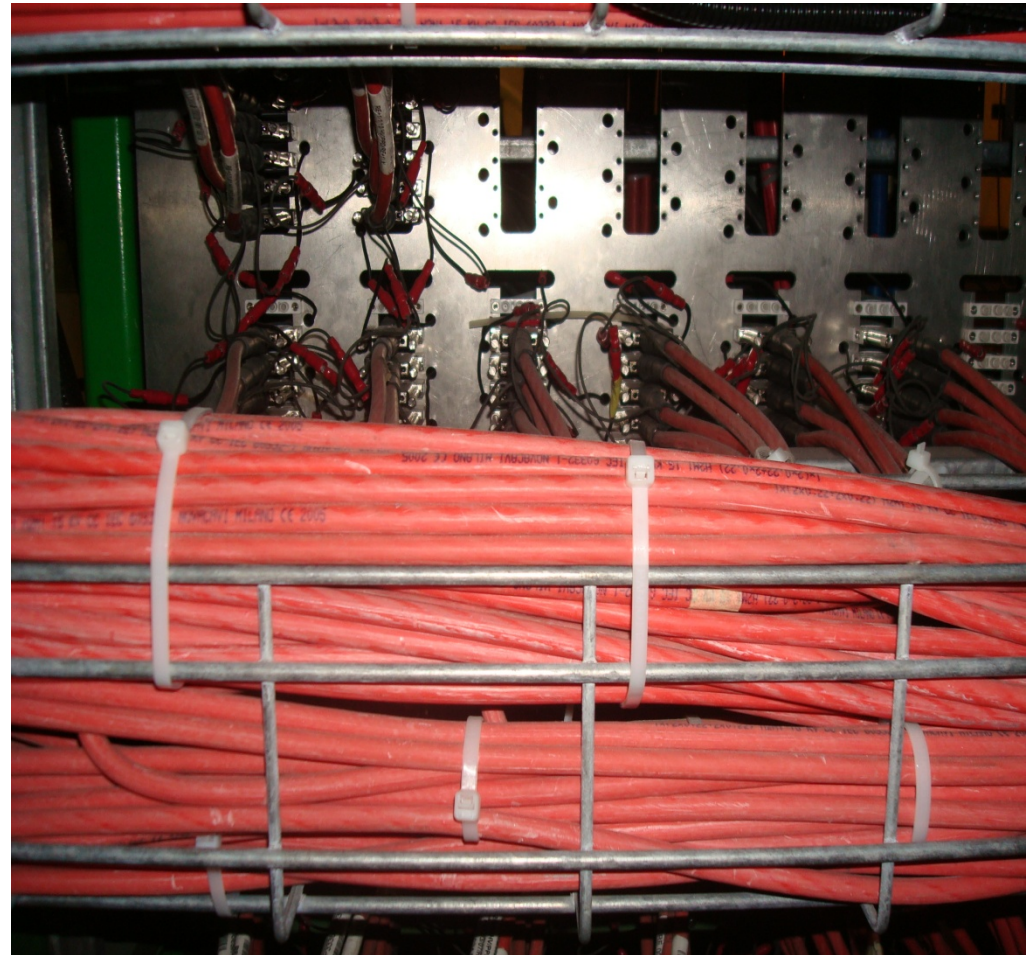
HV Cables connections to PP
