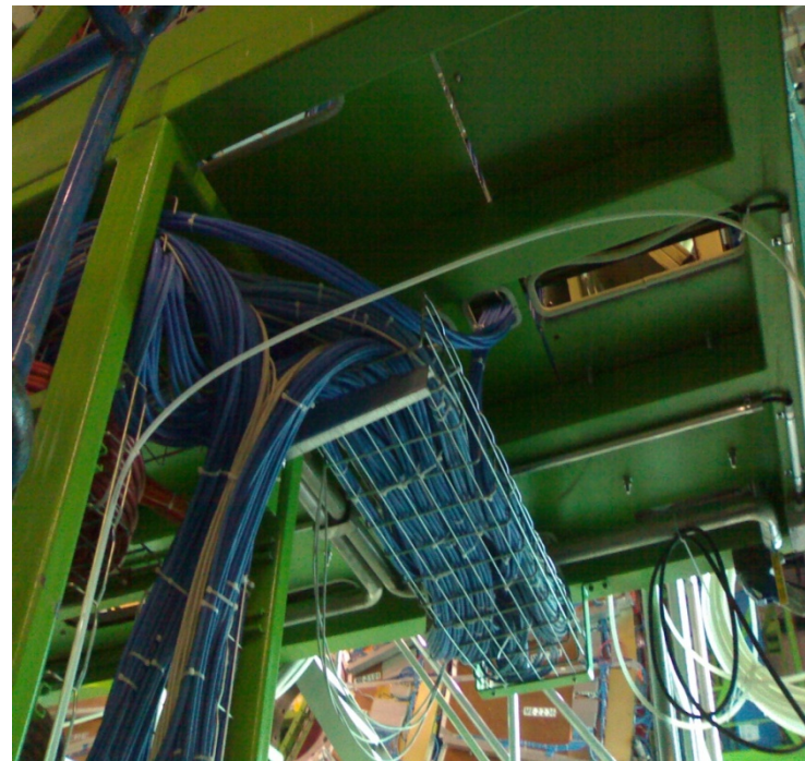
Signal + DCS cables in cable tray
