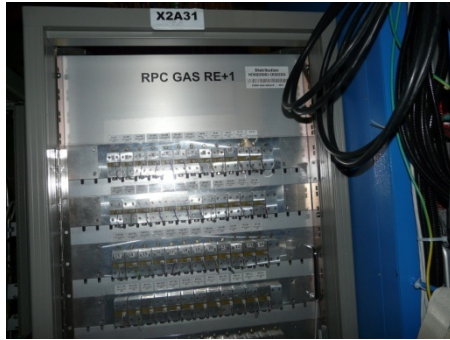
• Gas rack front
