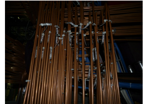
• Gas pipes from rack leading to disk
